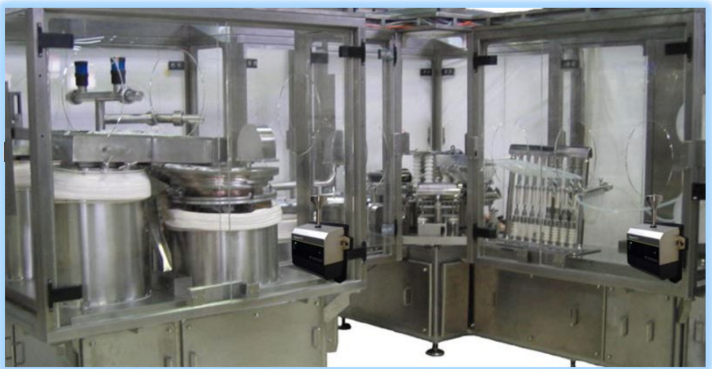
Filling machine being monitored with remote particle counters (with internal vacuum)
