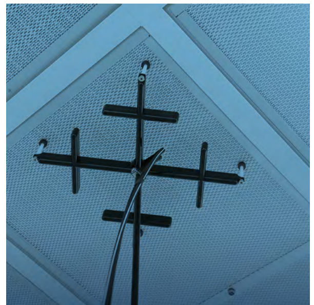
Fig 5.0 A HEPA filtered vent undergoing air velocity testing.
