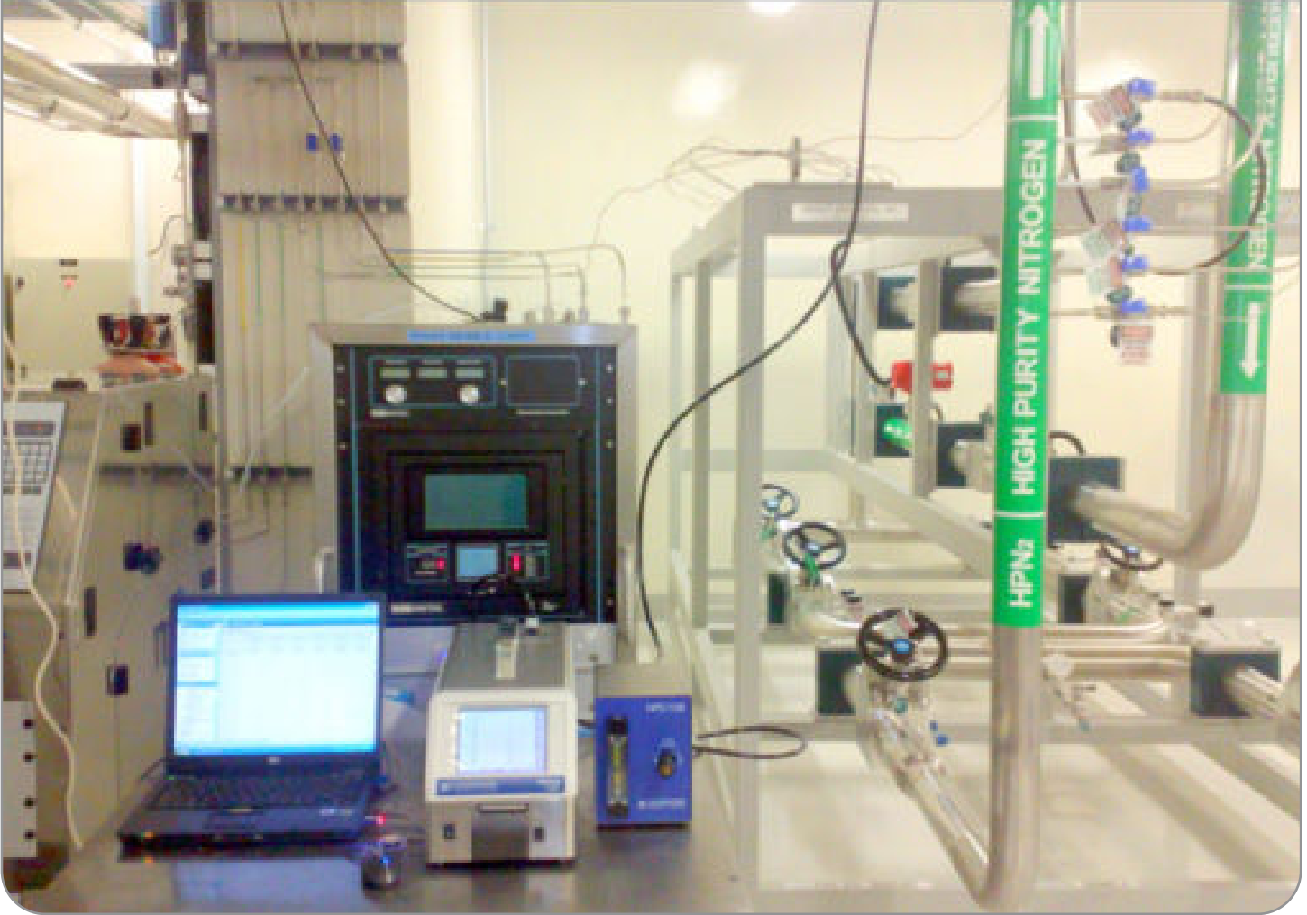
Application example of Semiconductor Nitrogen gas system being monitored down to 100nm
